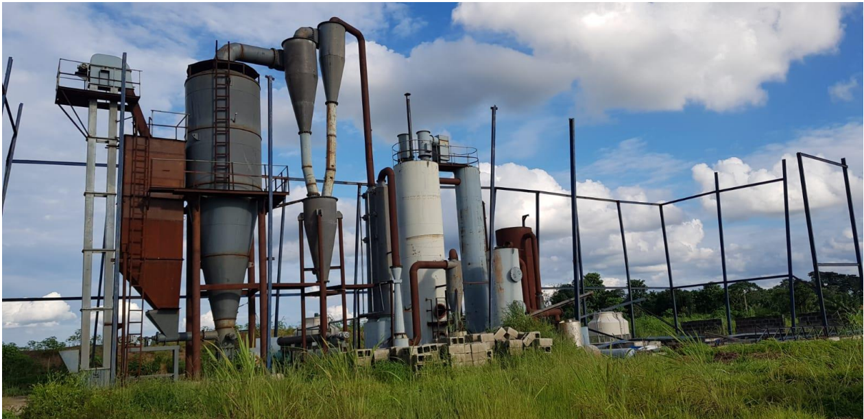
The main components on site are missing a protective rooftop
