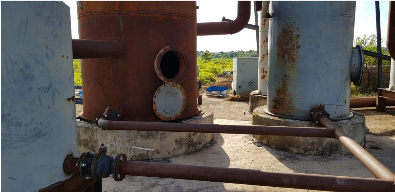
Corroded condition of vessel and pipework and missing flange bolts on Buffer Tank
