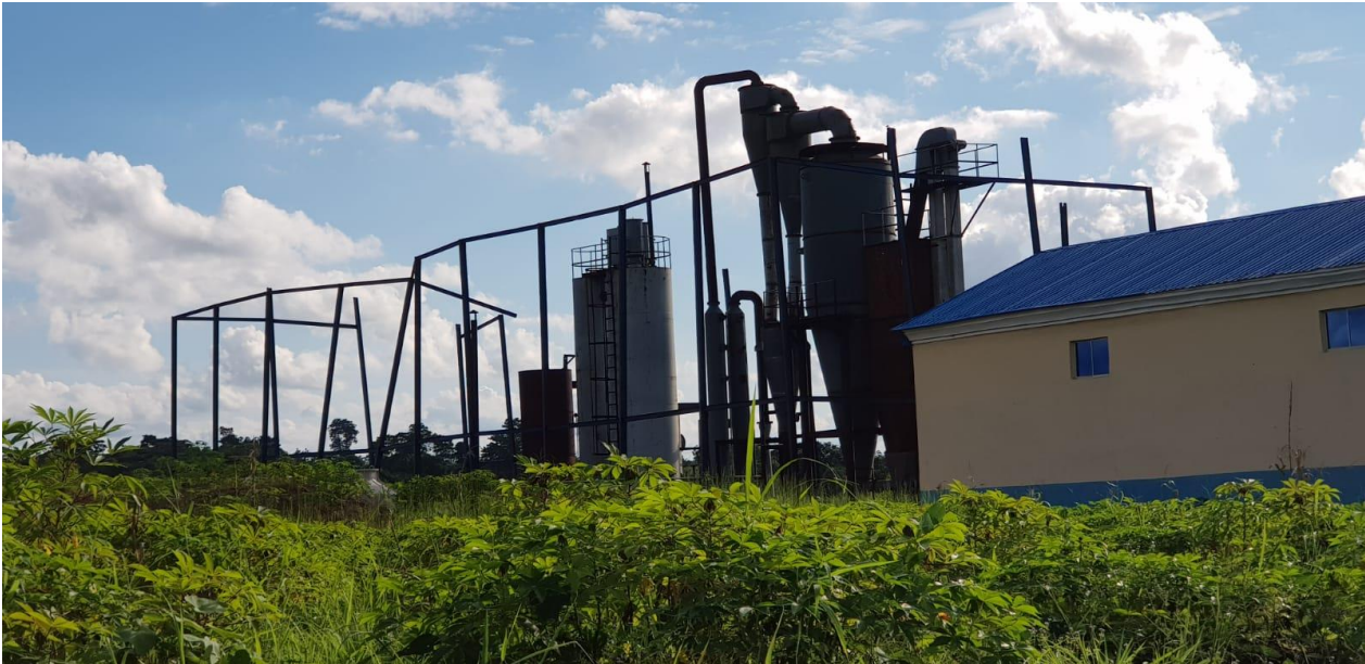
Overview of Ikwo site alongside rice husk storage and energy plant building
